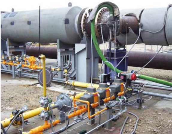
Figure 2: Gas Train in the Foreground Used to Fuel the Burner.
