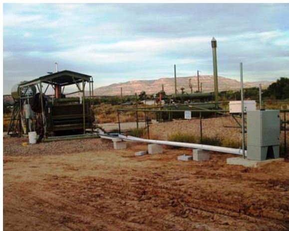
Figure 1: Emissions Sample Line Leading to the Enclosed Testo Emissions Analyzer.
