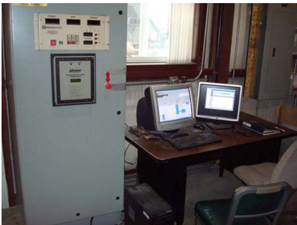
Figure 2: Data Acquisition System in the Control Room.
