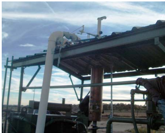
Figure 1: Emissions Sample Line Leading to the Stack.
