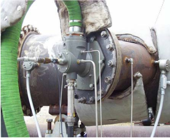
Figure 1: Low Emissions Burner Installed on the NGML Turbocharger Test and Research Facility.
