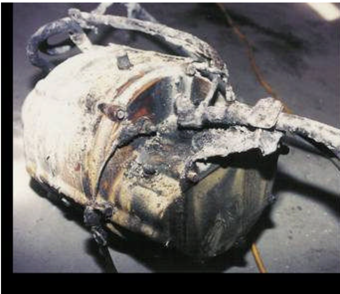
Photo 6b: 50-DN, Result of Failed B+ Stud Insulator
