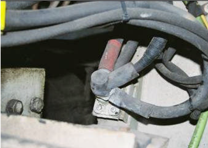
Photo 8a: Bulkhead Connection 50-DN
