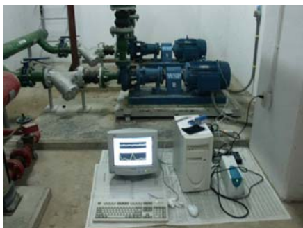
Condition monitoring of university plant equipment, ERM project
